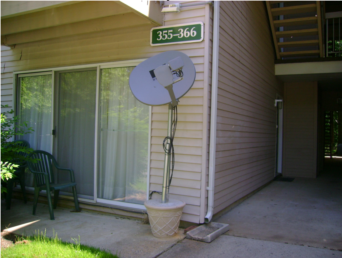
Conforming Satellite Dish Installation
